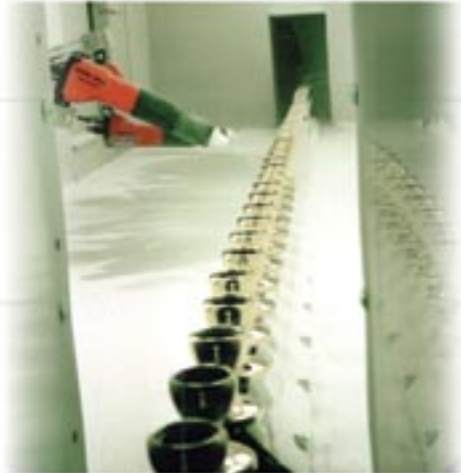
Booths for powder coating systems of all types – from door knobs to rail cars!
