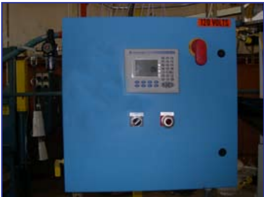
System Control Panel
